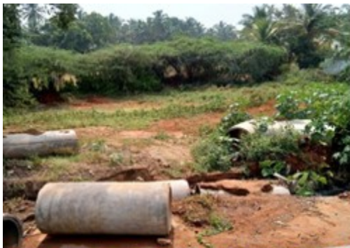
LIFT STATION-3 at Sundapalayam
